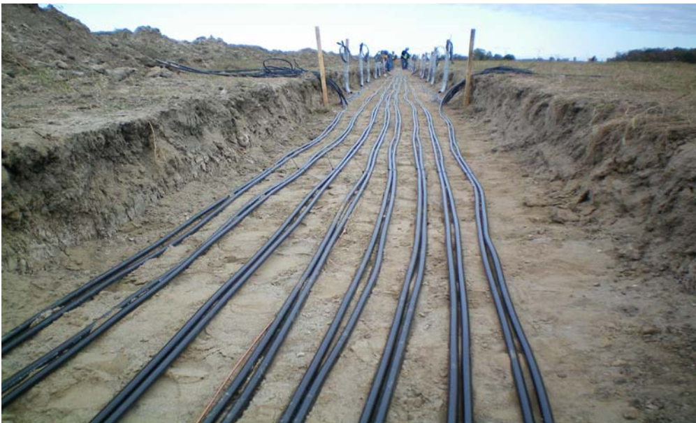
Photo Plate 12: Example of Cabling Being Installed in Trenches for Interconnection to Grid
