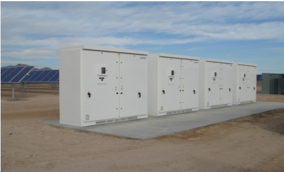
Photo Plate 8: Outdoor Compatible Commercial Inverters (Source: Xantrex)
